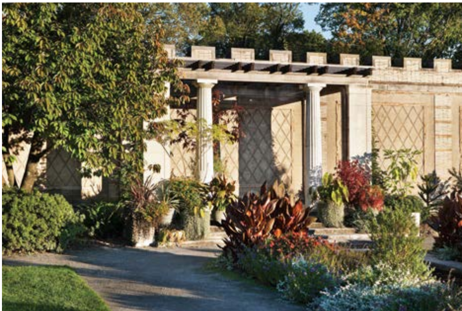
One of the columns in the East Stoa was recently repaired but retains an age crack. The plantings around it are new.
